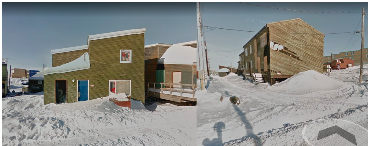
Pictures from Google street view (© 2013) in Iqaluit Left: Cracks in structure, windows shifted within frame Right: Structure in state of disrepair, no windows. Unit is likely uninhabited, but the other unit in the duplex seems to be occupied. Many other buildings have no windows, only plywood.
